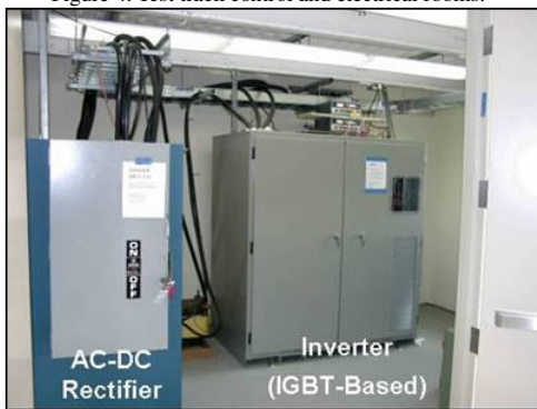
Figure 5. Electrical room interior view.
